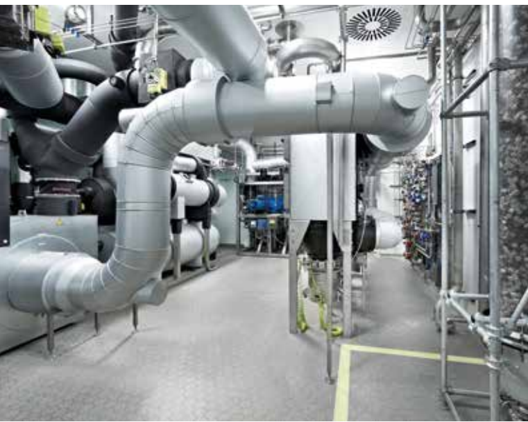
Technical area of a coating system with nitrogen circuit and solvent condensation
